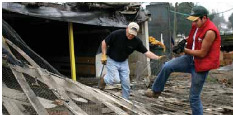
John Raumann (left) and Michael Mauel (right) tear off the chicken wire from the demolished fruit stand.
