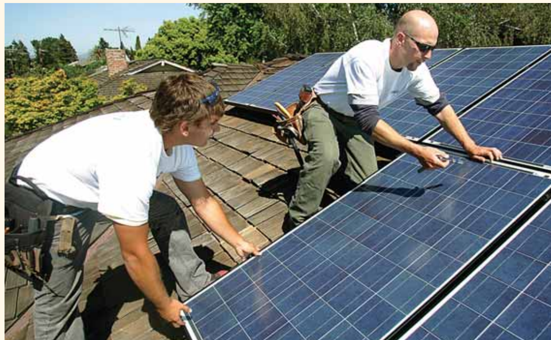
SolarCity workers Ivan Shynhel (left) and Mike Smith secure photovoltaic panels on the roof of Paul McGruder's home on Wasatch Drive.
