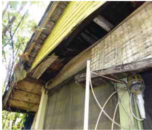
City inspectors documented the decay at Loretta Pangrac's house before it was demolished.
