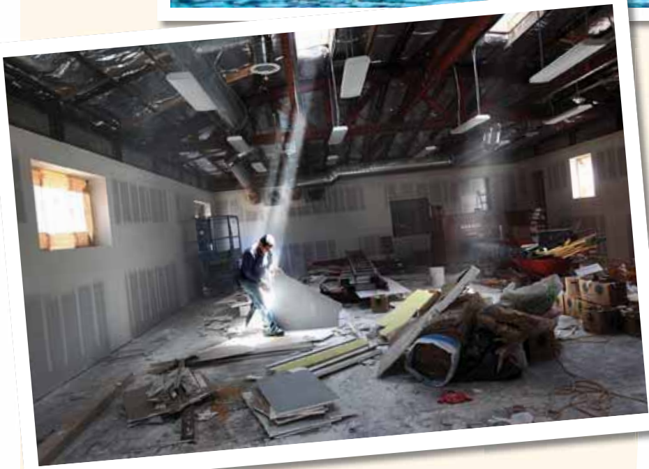
Jose Oriana sorts through drywall during construction on Mountain View's new Dayworker Center on Escuela Avenue.
