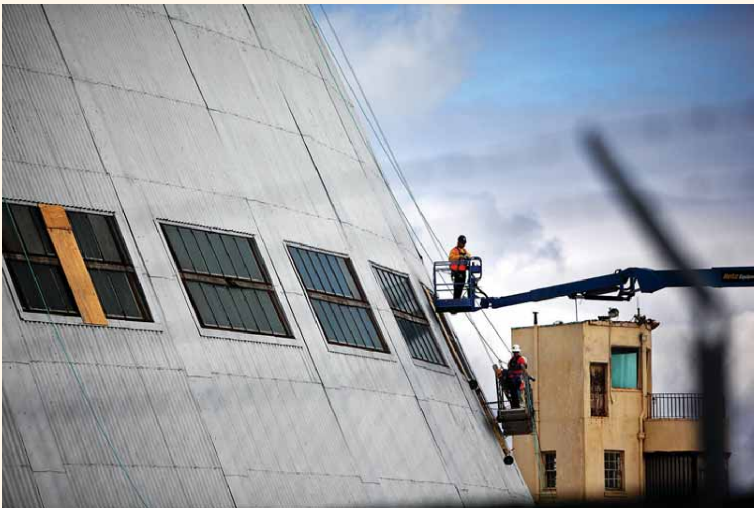
Crews earlier this week worked to prepare Hangar One, a 200-foot-tall hangar built during the Depression, for the project. MICHELLE LE
