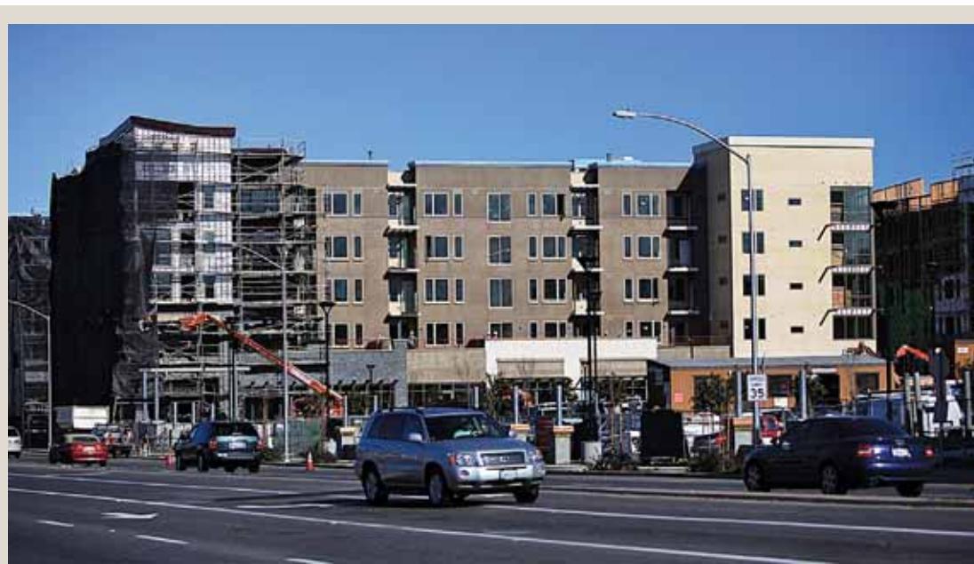
Construction is going quickly in the first phase of Merlone Geier's project at San Antonio Shopping Center.
