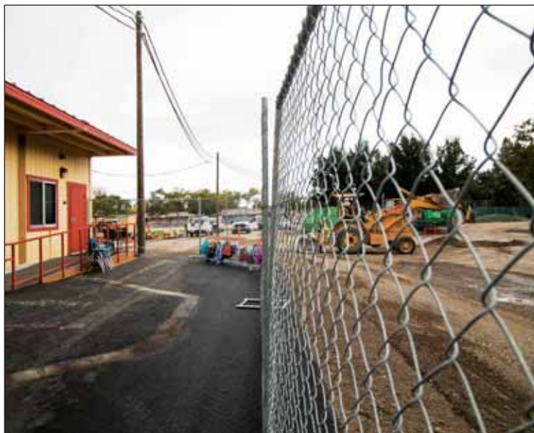
Brightly colored backpacks are hung on a fence separating classrooms from the construction site at Stevenson Elementary School.
