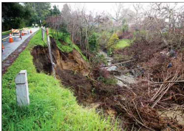
This photo from Jan. 18 shows the initial damage to the creek bank along the segment of Stevens Creek Trail between El Camino Real and Yuba Drive.
