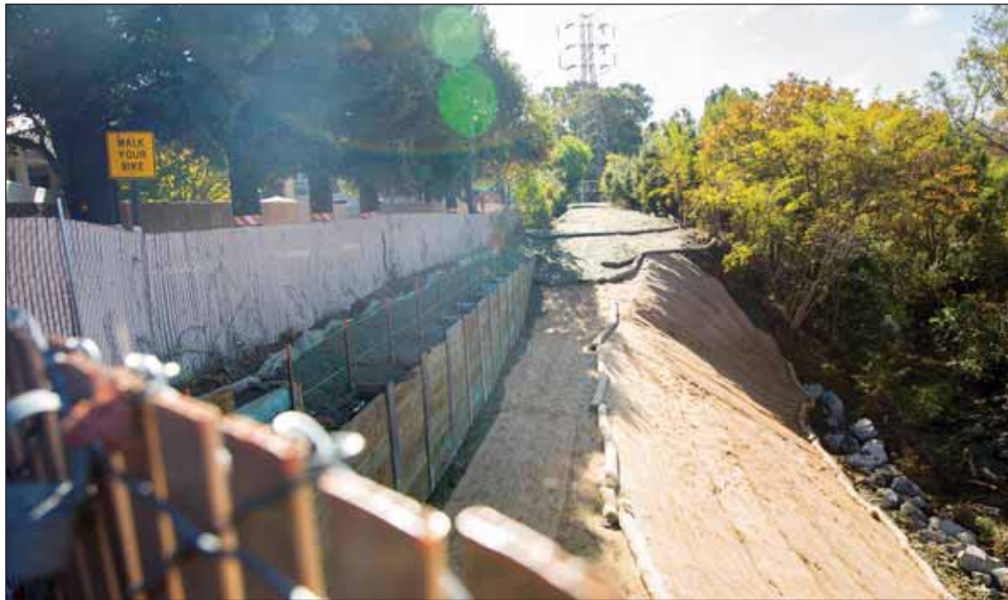
The $500,000 repair job should prevent further erosion to the creek bank until permanent repairs can be made next year.
